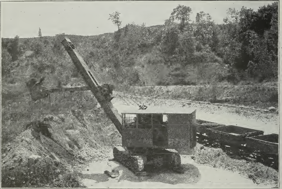
Fig. 20. Gasoline tractor shovel and side dump cars used for removing overburden at the quarry of the Wedron Silica Company. In the background is a cliff of St. Peter sandstone capped by glacial drift. (Photograph by courtesy of Wedron Silica Company.)
